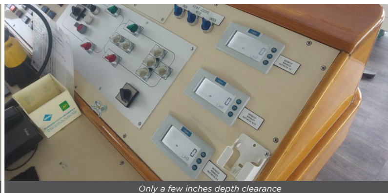
Only a few inches depth clearance
